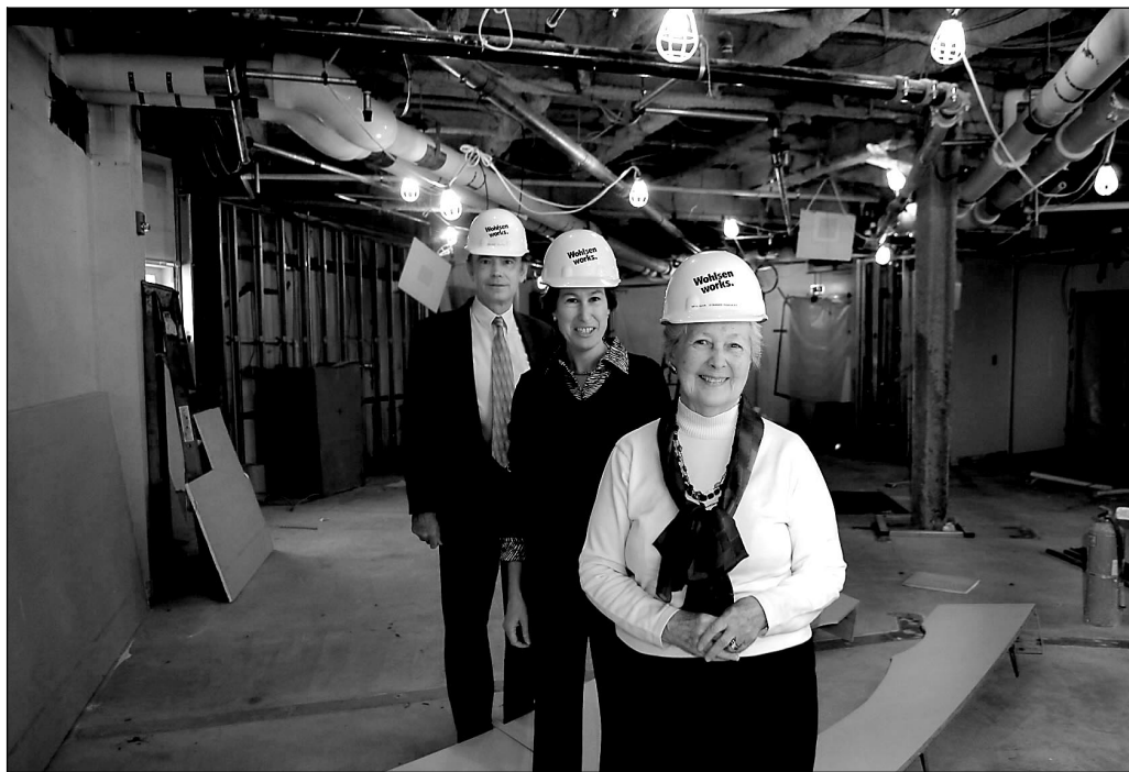
Mary Barton, a member of the board and the renovation committee; Ann Brooke, who is helping lead the capital campaign; and Brant Hart, executive director (front to back), stand where a new dining room will be built as part of a $23 million renovation.
